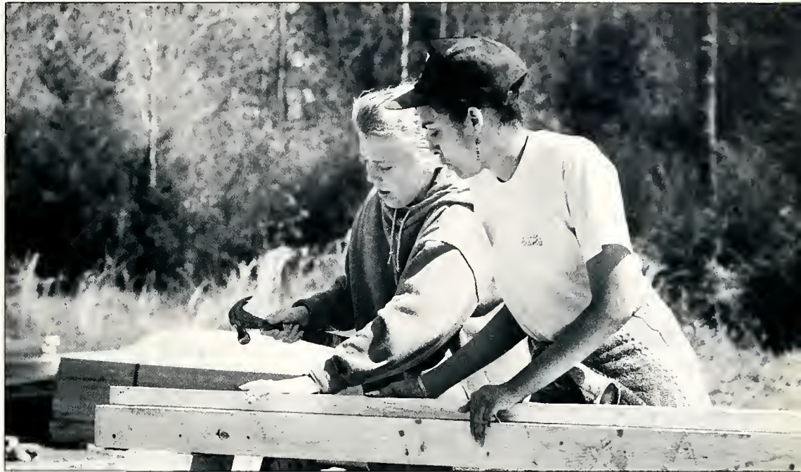
Nancy Zehl '94 and French instructor Marie-Christine Lagier work on door frames. Although she didn't bring many building skills, said Zehl, she brought what is most important: "All you need is an ability to care."
