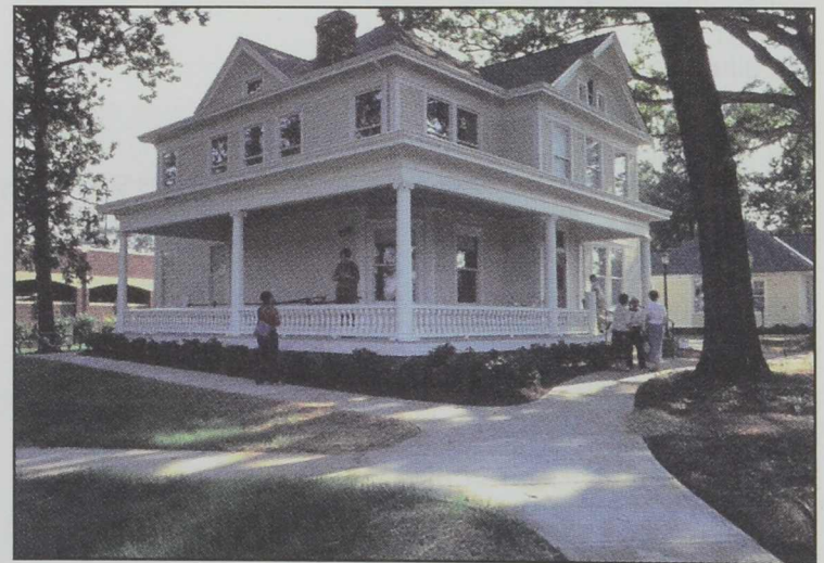
GARY W. MEEK PHOTOGRAPH Students check out the renovations at 124 E. College Ave. The house once played host to legendary crooner and movie star Bing Crosby.
