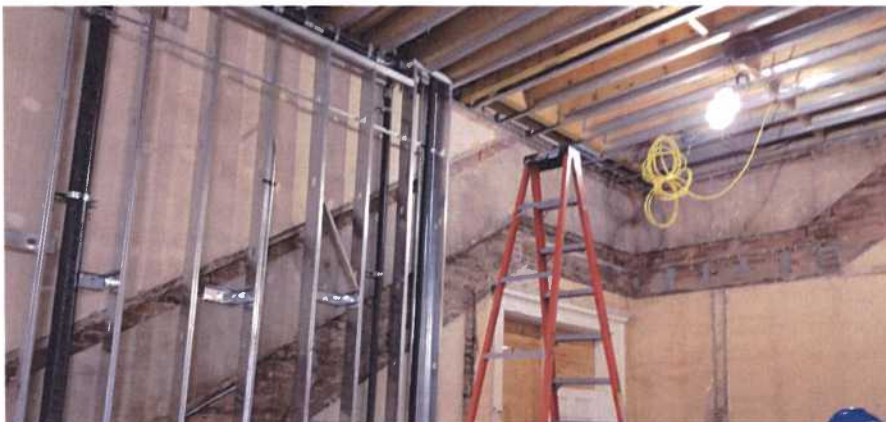
The gutted first floor staircase. Photo courtesy of Karina Leung '18.
